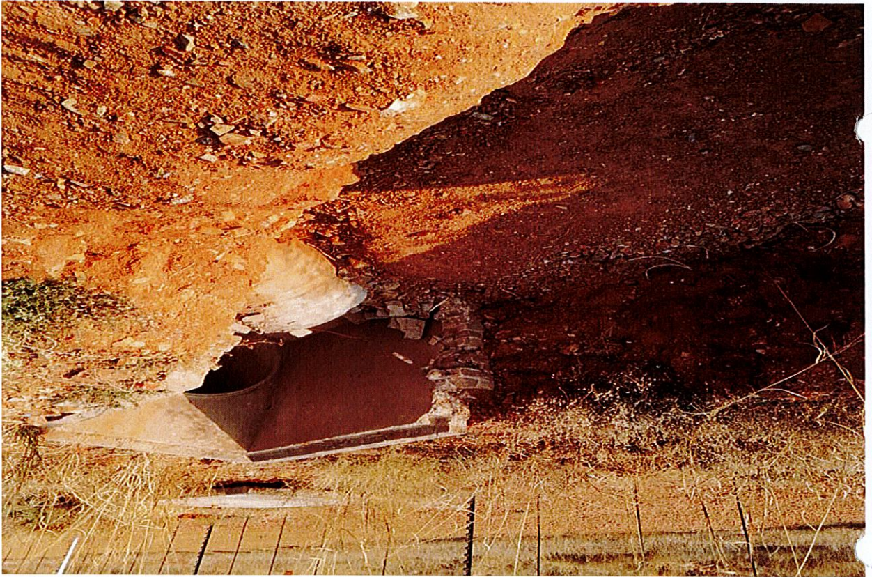
Figure 28 EXTENSION 6 PHASE 3 AND 4 STORM WATER BY MPAC RESEARCHER
