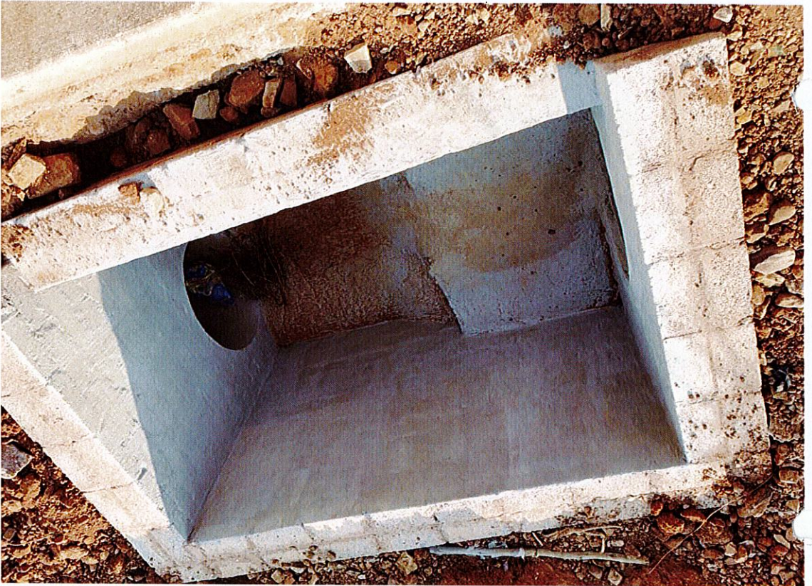
Figure 29 EXTENSION 6 PHASE 3 AND 4 STORM WATER BY MPAC RESEARCHER
