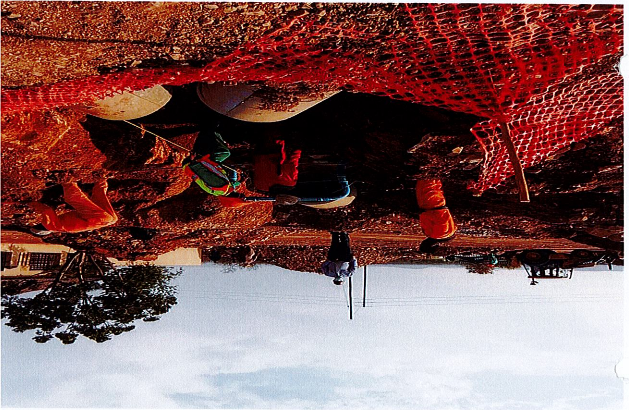
Figure 30 EXTENSION 6 PHASE 3 AND 4 STORM WATER BY MPAC RESEARCHER
